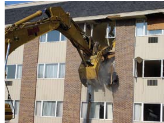
Demolition begins to make room for the new Town Center at The Holmstad
